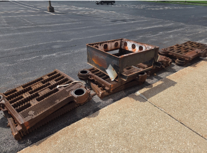
Close up of single boiler with cover removed
